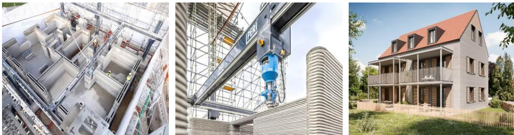
Figure 6. BOD2 3D printer by COBOD company was used for the construction of building in Wallenhausen [11]
