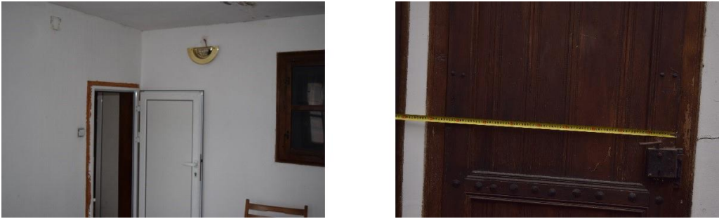
Figure 4. The current state of the doors
