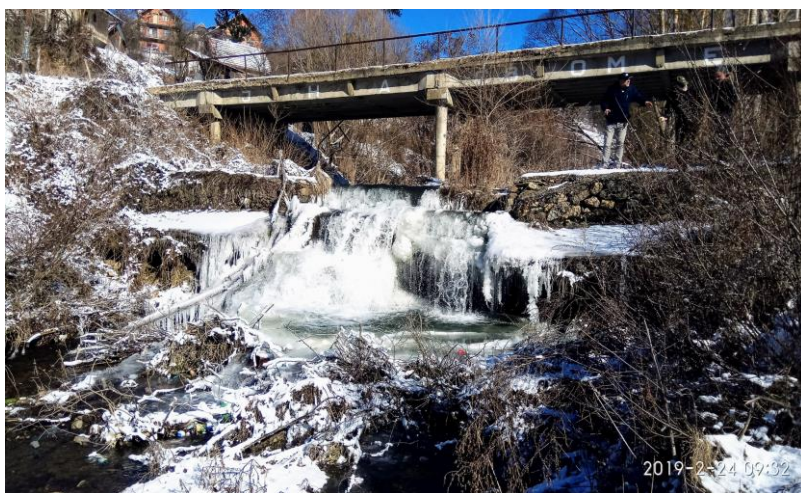
Figure 2. The bridge on the Tripušnica river in the village of Radovnica during winter
