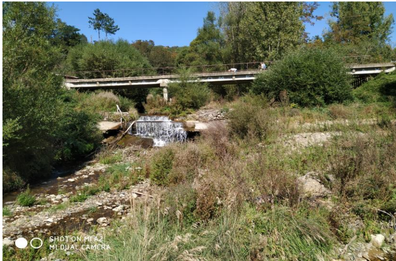
Figure 1. The bridge on the Tripušnica River in the village of Radovnica during summer
