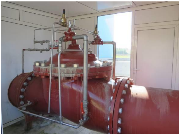
Figure 2b. The synchronous outlet valve itself
