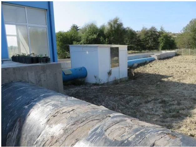
Figure 2a. The branch and powerhouse of the synchronous valve
