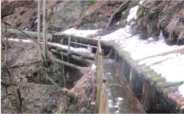
Fig. 2. Steel penstock protected by logs from rock-fall
