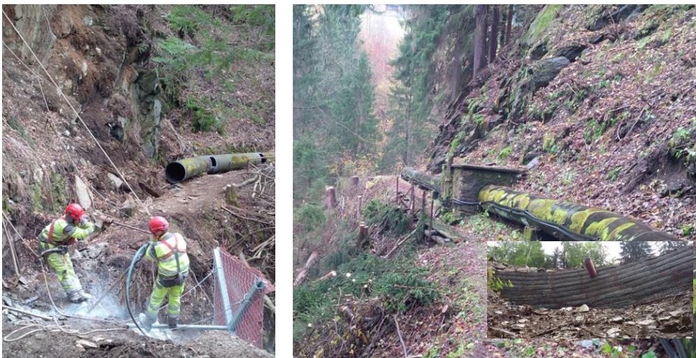
Fig. 7. Penstock before / while dismantling; installation of slope support system; reinforced earth at access road
