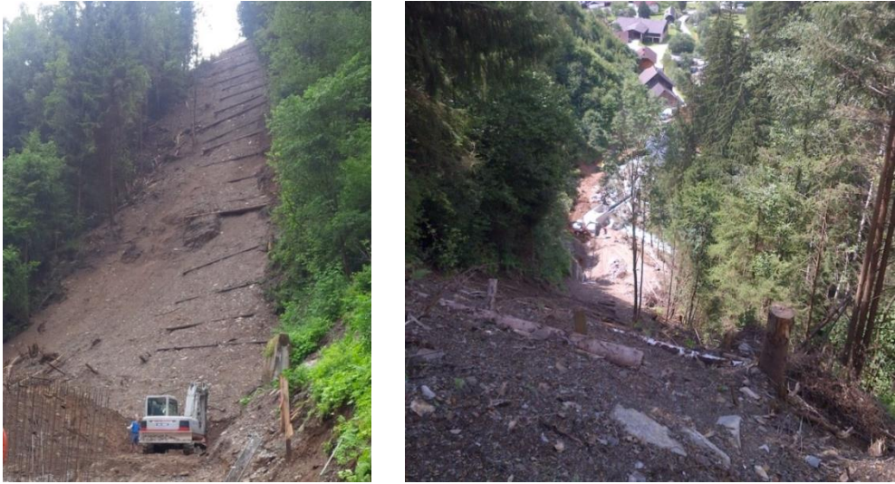
Fig. 11. Steep slope section of the penstock before hydro seeding; hydro seeding machinery
