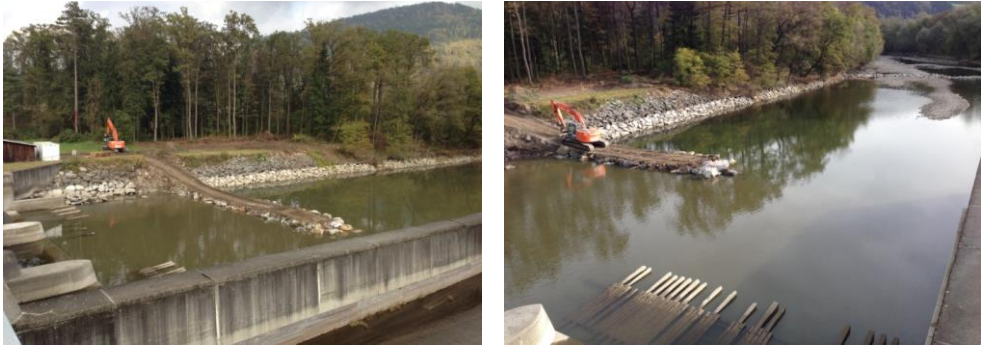
Fig. 5. Downstream scour backfill at the energy dissipation area of weir bay#1and #3 and sluice bay (source: VERBUND)
